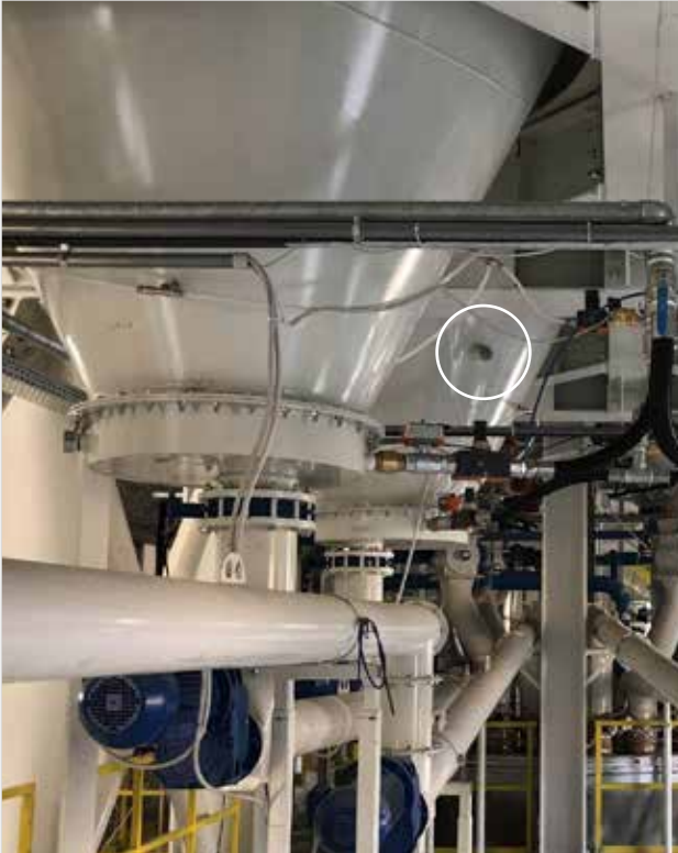
VBS (aireadores) - Silos
